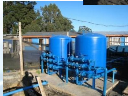
Potable Water Storage
